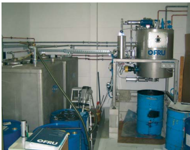
Recycling plant ASC-150.
