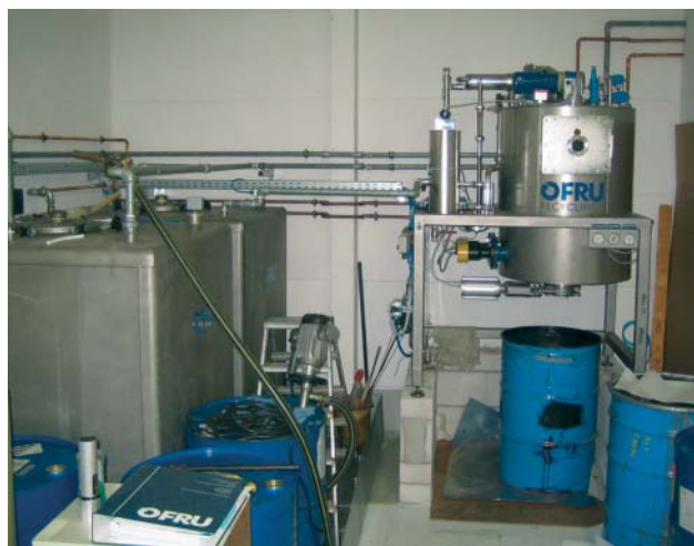
Recycling plant ASC-150.
